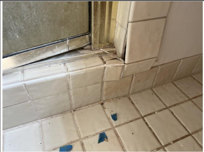
12. HM#3: Bathroom tile/grout/caulk
